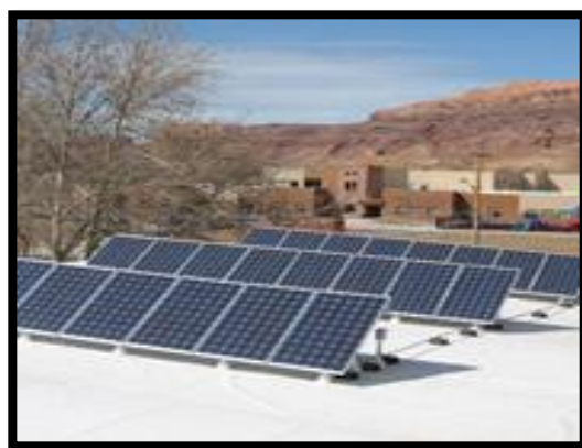
Figure 20. Moab Recreation and Aquatic Center Rooftop Solar
