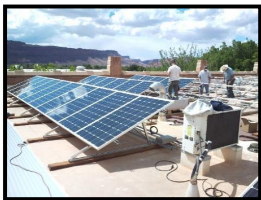
Figure 19. Moab City Center Solar Installation
