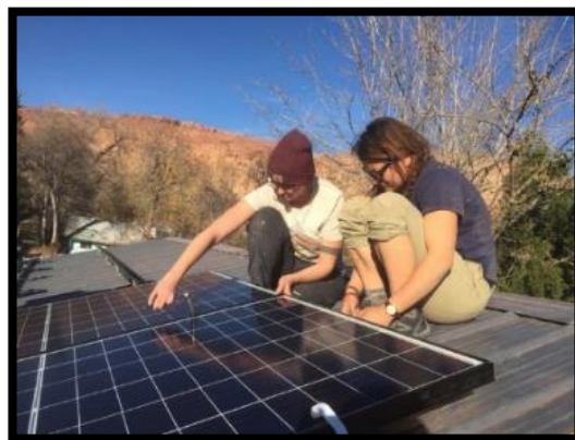
Figure 22. Community Rebuilds Solar Project
